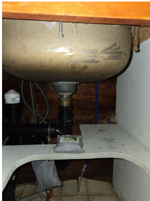
Picture 2: Under side of the kitchen sink. The glaze contains 1% chrysotile asbestos.
