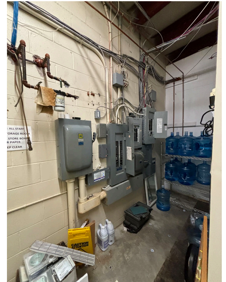
Existing Electrical Service Distribution
