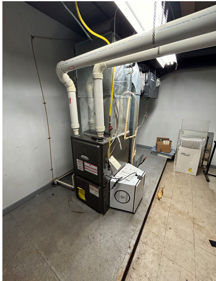
Existing HVAC Unit
